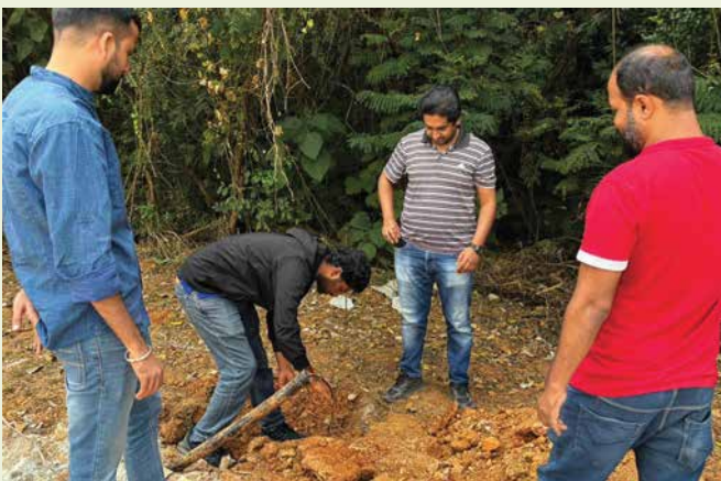
Rahul Nair (second from right), along with staff members from TINA and other vendors, inspecting a dug-out optic fibre cable outside the Division of Interdisciplinary Sciences building
