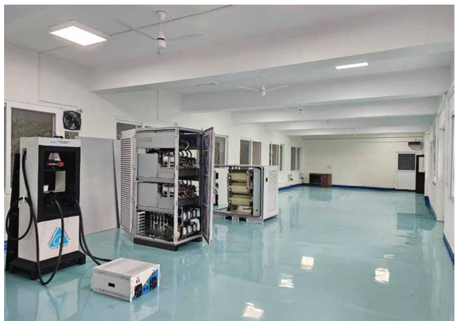
Upcoming 2,000 sq ft lab (11kV, 500-kW) under development at the Department of EE, IISc, in collaboration with Delta Electronics, which is being designed to test 500-kW power converters
