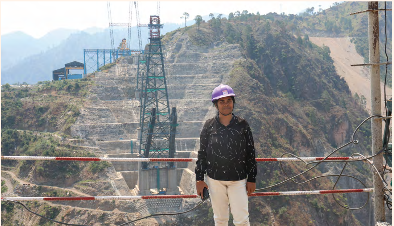
Madhavi on site at the Chenab railway bridge project, Jammu and Kashmir
