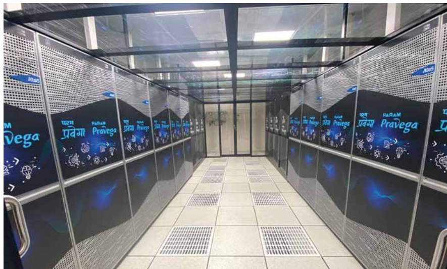
The supercomputer at the Supercomputer Education and Research Centre (SERC), IISc
