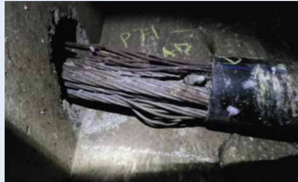
Picture showing the broken cable inside the bridge near Peenya
